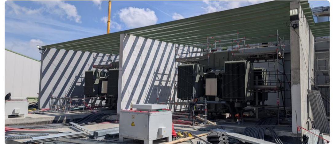
Substation transformer terminations
