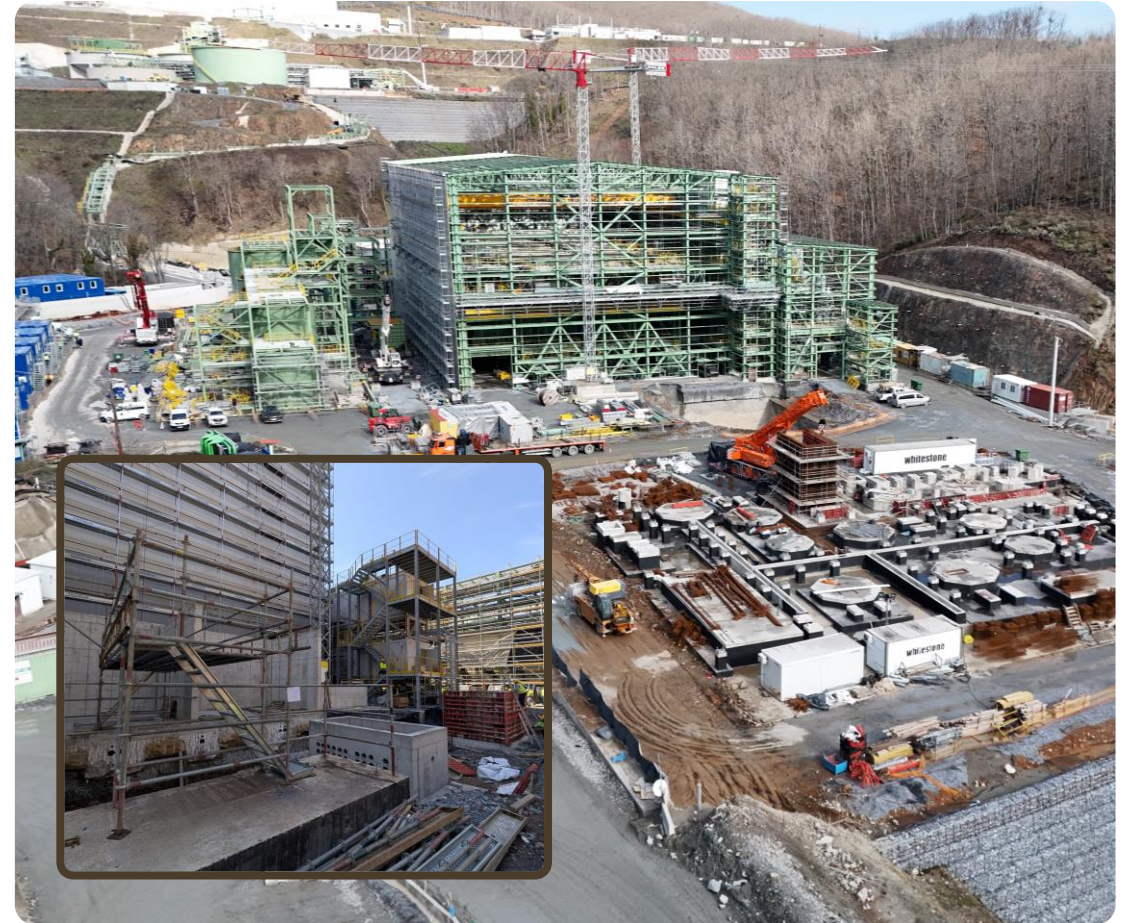
Tailings filter press building. Bottom left insert – closer up view of filter building pull pits.
