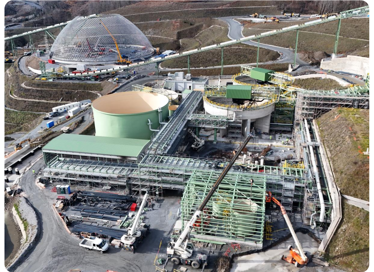
Tailing thickener pipe rack and distribution box
