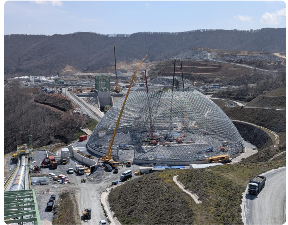
Primary crusher, dome and reclaim feeder
