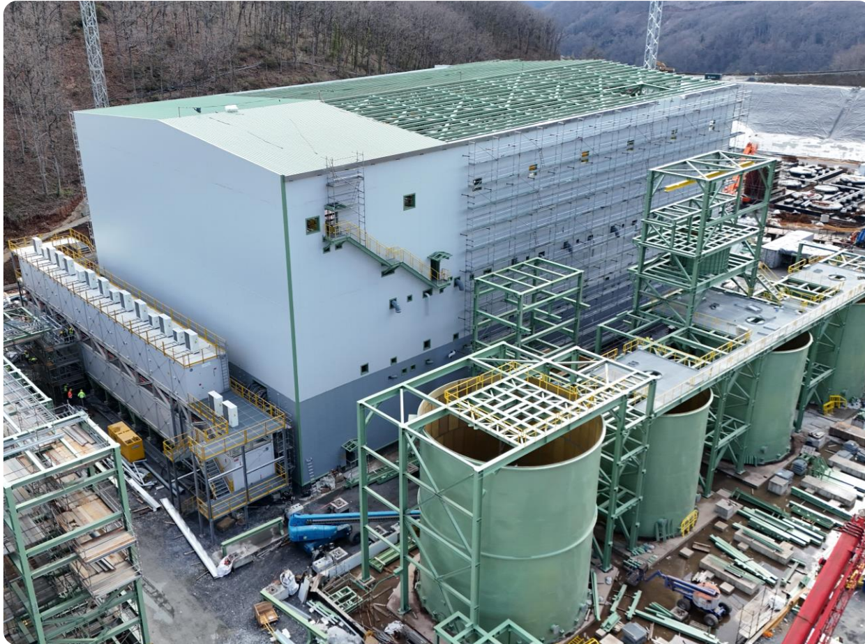
Filtered tailings plant overview, with tank farm progressing shown in front and the foundation of the compressor building on the left
