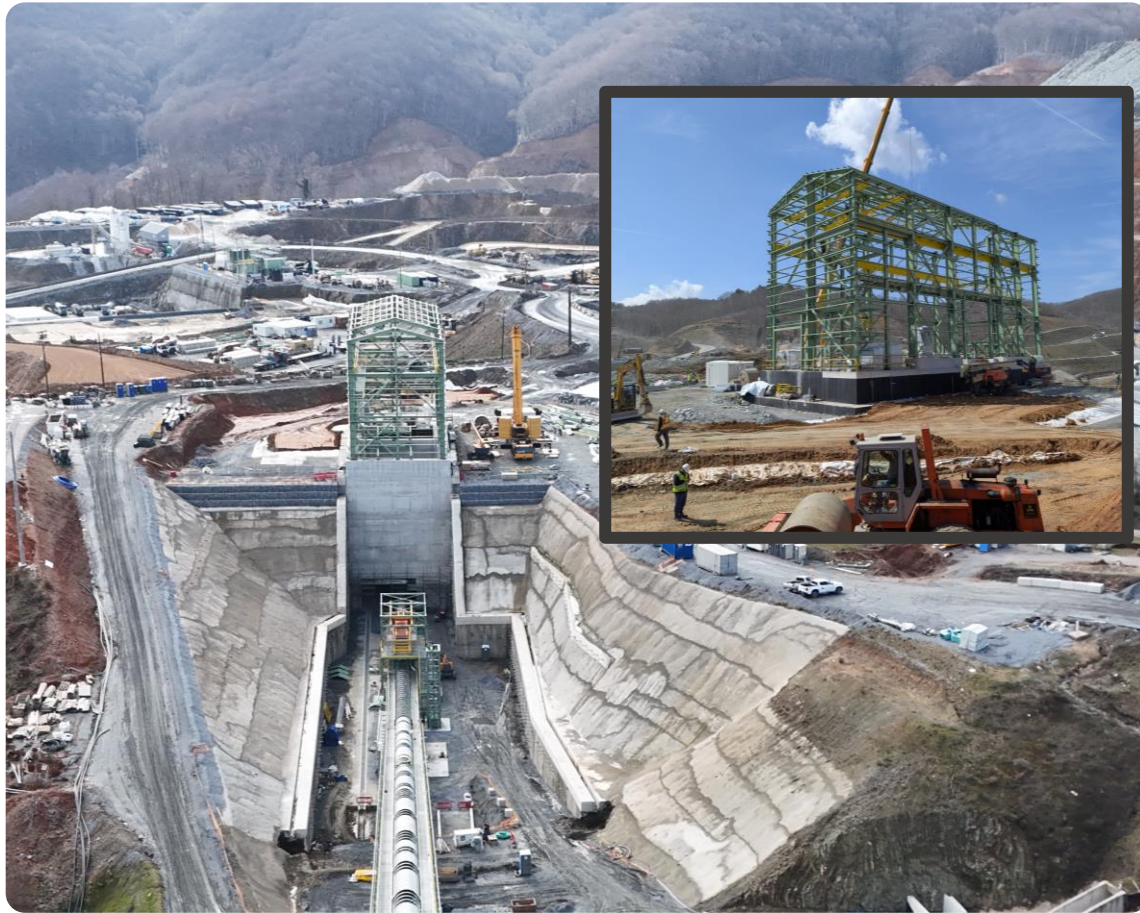
Primary crusher overview. Top right insert – closer up view of primary crusher building erection.
