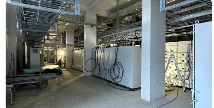
First Floor Electrical Room
