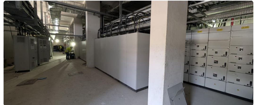
First Floor Electrical Room
